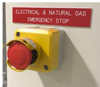
Figure 1 Example of electrical emergency stop red button.
